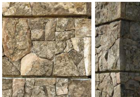
STONE VENEER - Montana Moss Rock natural stone dry-stack lay-up. Stainless steel masonry anchor system.
