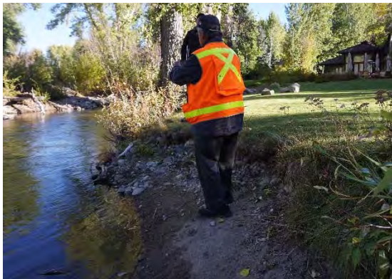
Figure 1: Eroding channel bank in project transition area.
