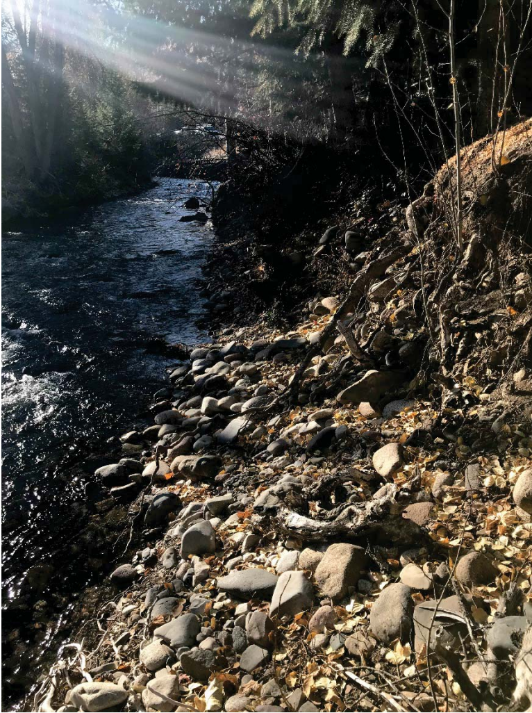
Figure 1: Overhanging bank, exposed tree roots and loose bank material
