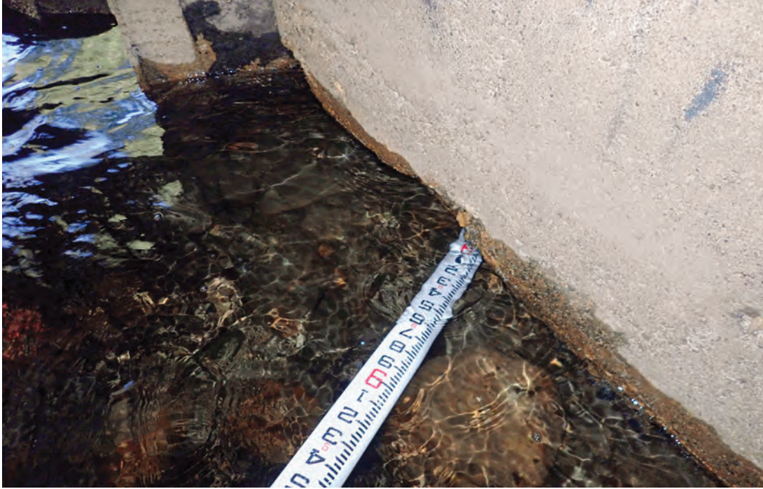
Undermining at northeast corner looking northeast.
