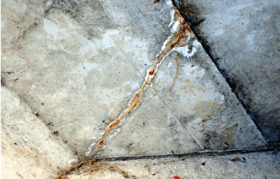
Cracks in flanges at east abutment.
