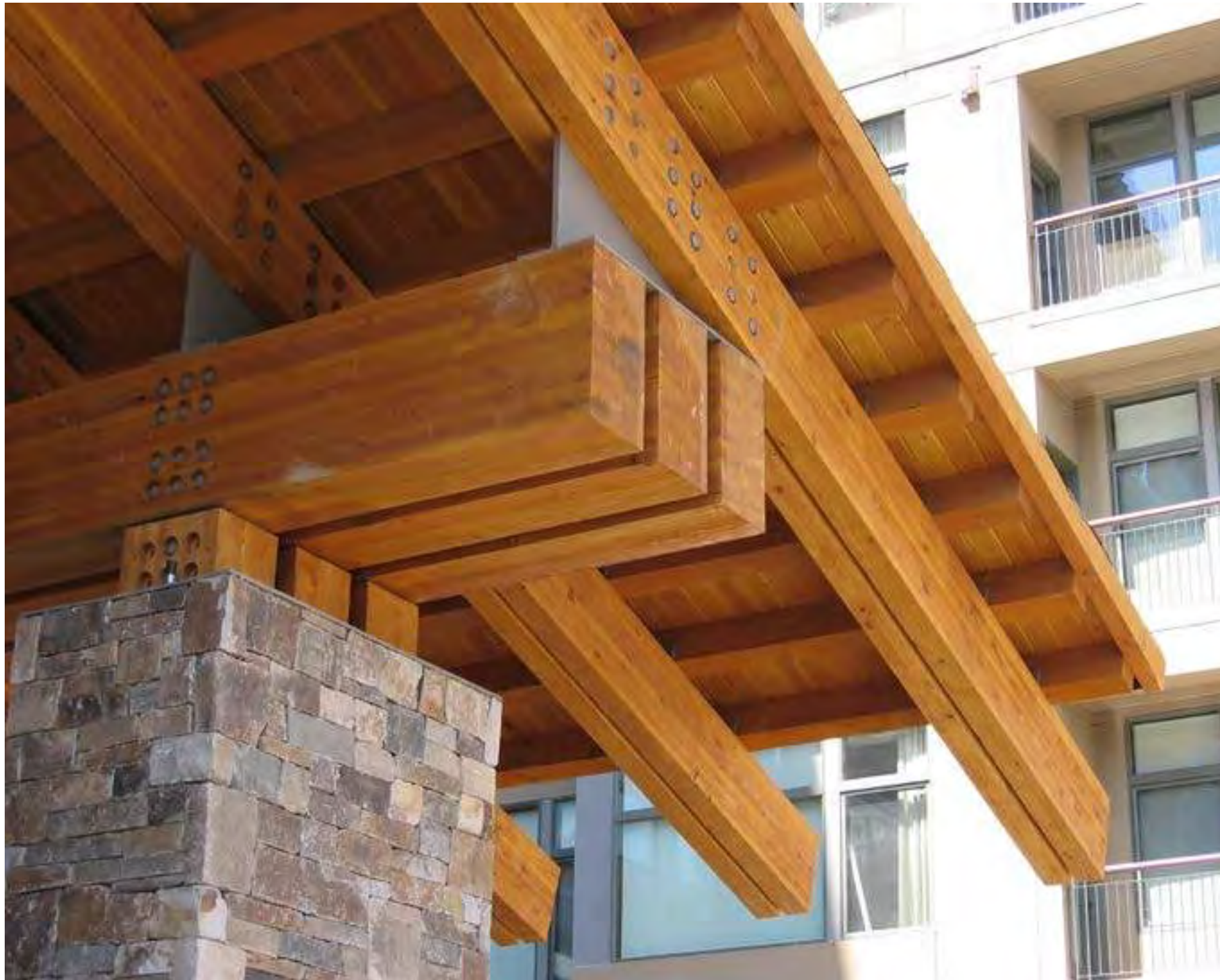
HEAVY TIMBER GLULAM BEAMS, RAFTERS AND COLUMNS with painted galvanized structural steel knife-plate connections. Fasteners to be recessed galvanized steel or stainless steel. Clear heart Western Red Cedar heavy timber purlins and T&G decking with resawn finish. Wood clear coat stain.
