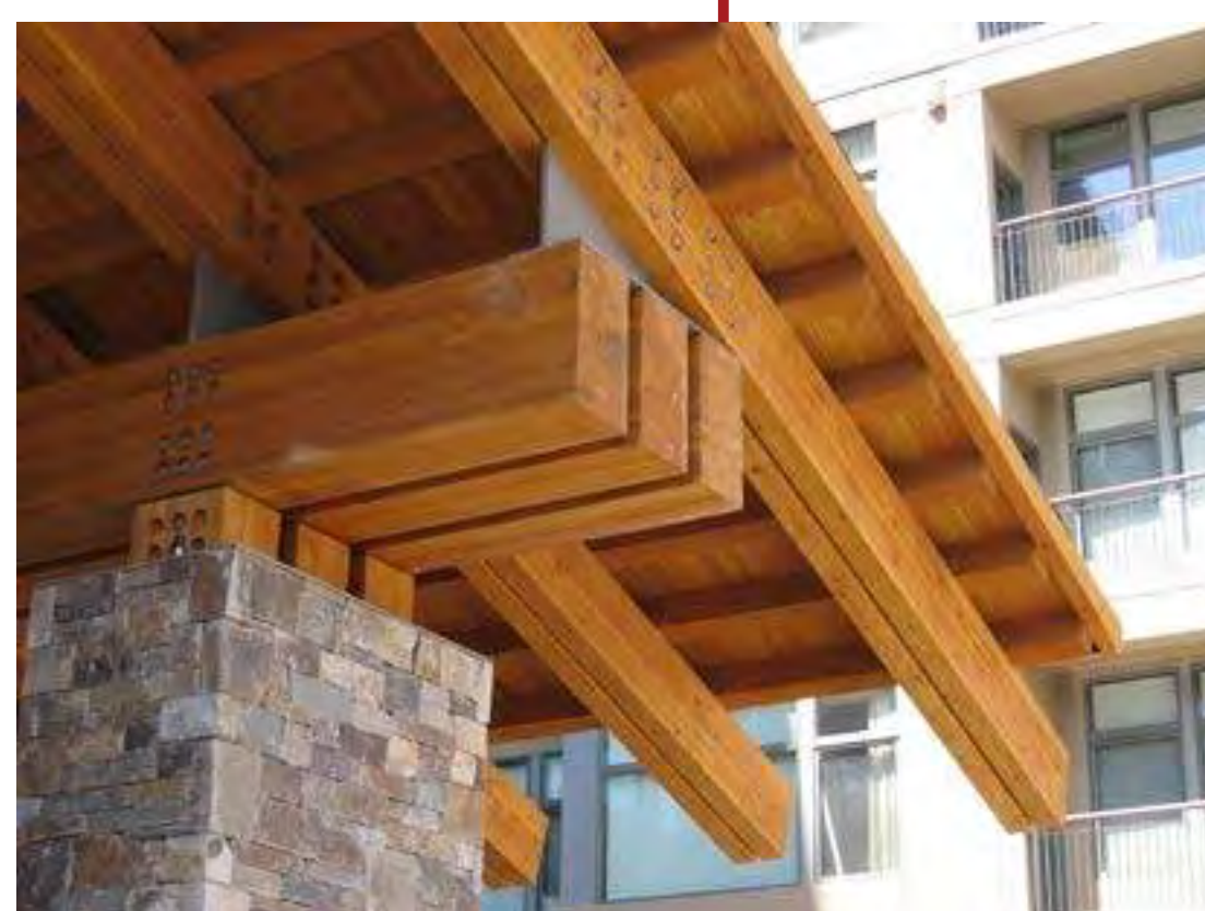
HEAVY TIMBER GLULAM BEAMS, RAFTERS AND COLUMNS with painted galvanized structural steel knife-plate connections. Fasteners to be recessed galvanized steel or stainless steel. Clear heart Western Red Cedar heavy timber purlins and T&G decking with resawn finish. Wood clear coat stain.
