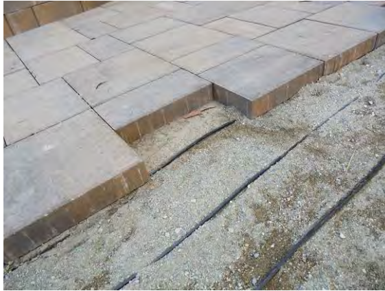
Pavers with radiant snowmelt system integrated.
