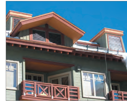
Group and screen mechanical units from view.
