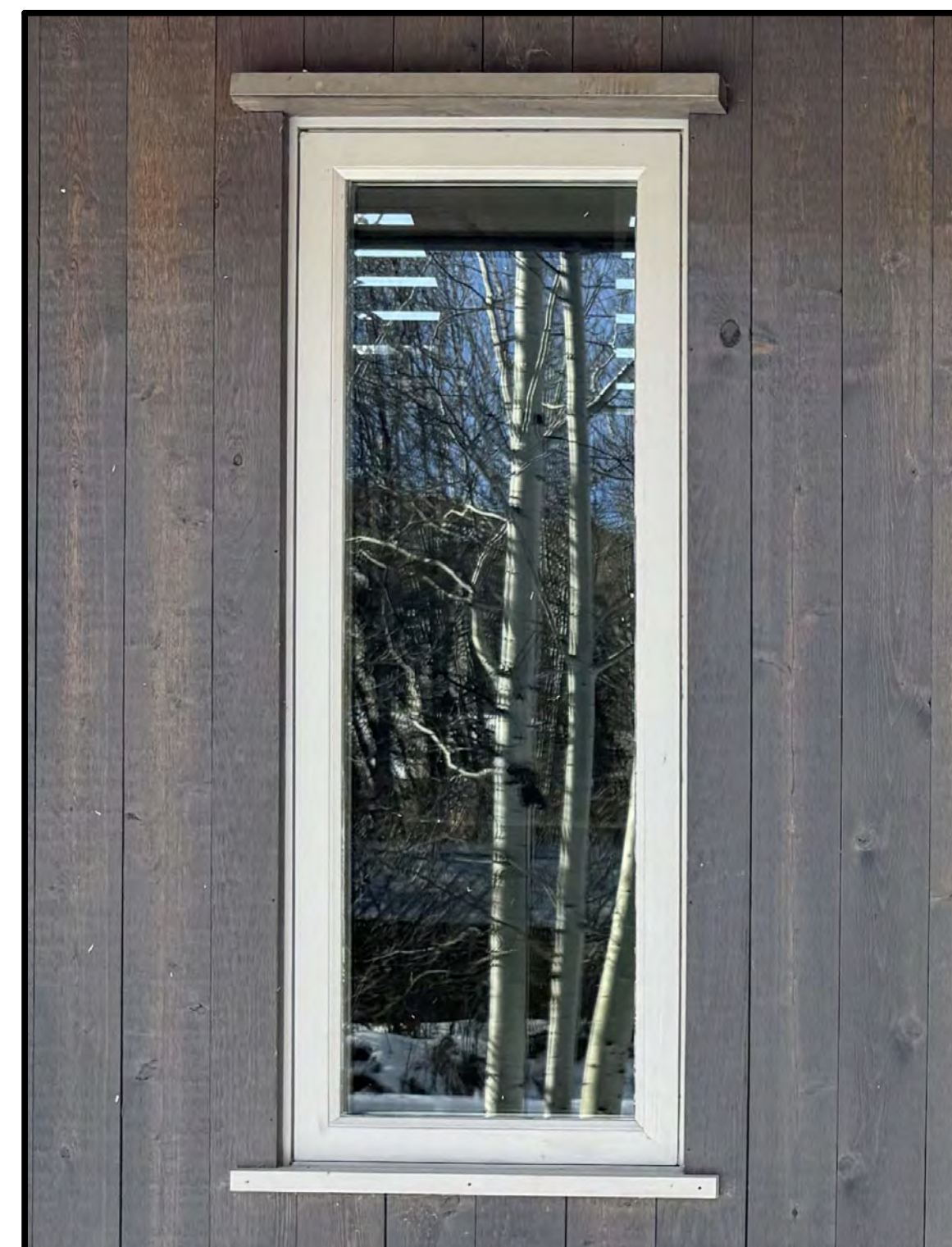
WINDOWS EXISTING EXTERIOR MATERIAL PROPOSED WINDOWS TO MATCH EXISTING ALUMINUM CLAD WOOD WINDOWS
