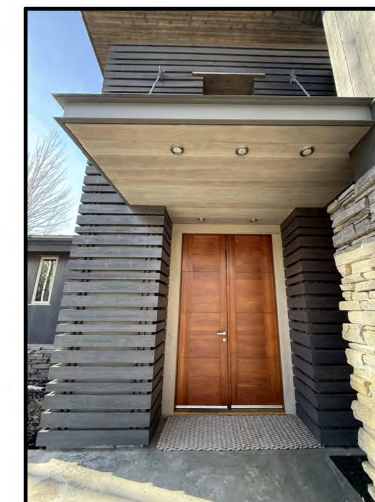
EXTERIOR LIGHT A LIGHT TYPE - EXISTING RECESSED CAN LIGHTS UNDER ENTRY CANOPY DARK SKY COMPLIANT
