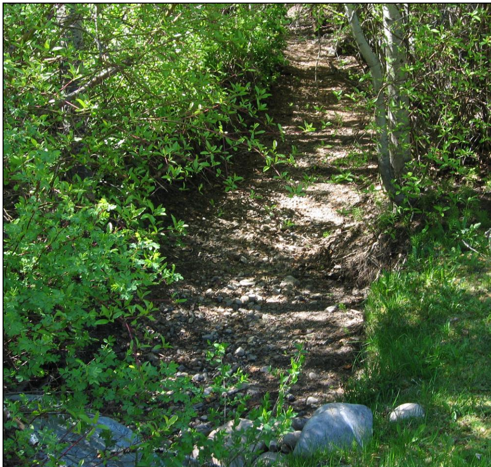
Figure 15b. Reinheimer Canal also known as Bowcut's Ditch was built in 1883. Digital Image GEM 5 # 36, view north.
