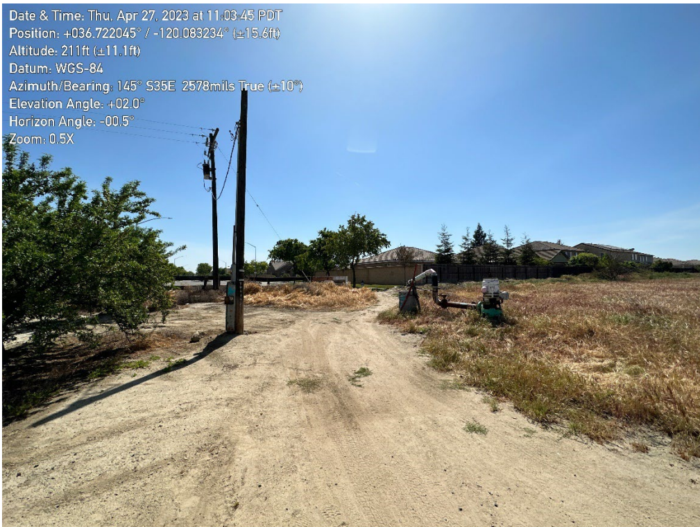
Photograph 4: View of two pole-mounted transformers and an irrigation well located on the northeast corner of the subject property.
