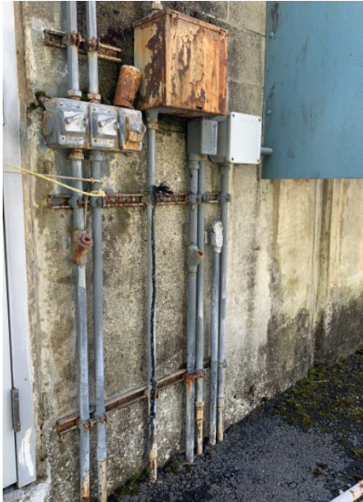
9. Switches & Conduits show heavy corrosion at exterior wall mounts.
