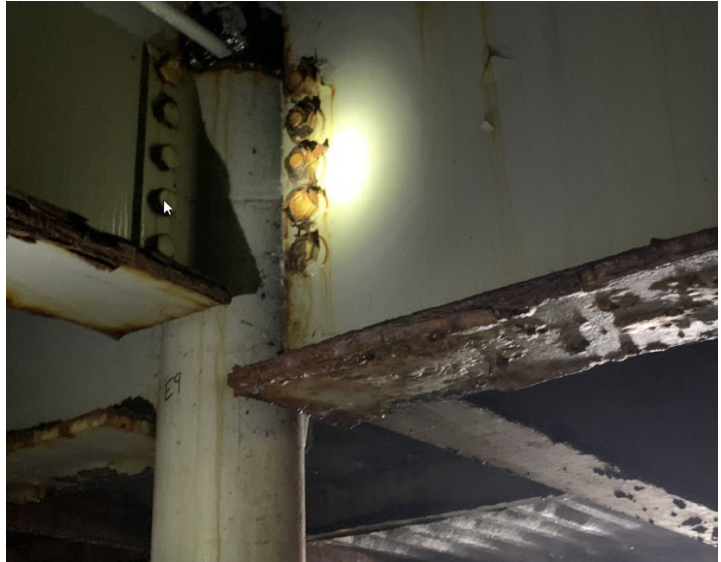
10. Corrosion at connecting bolts. This is the central 9" diameter support column for the roof between the two effluent tanks.
