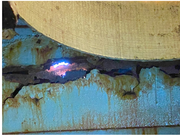
4. Corrosion of metal framing at the roof vent exhaust opening. Note daylight showing.
