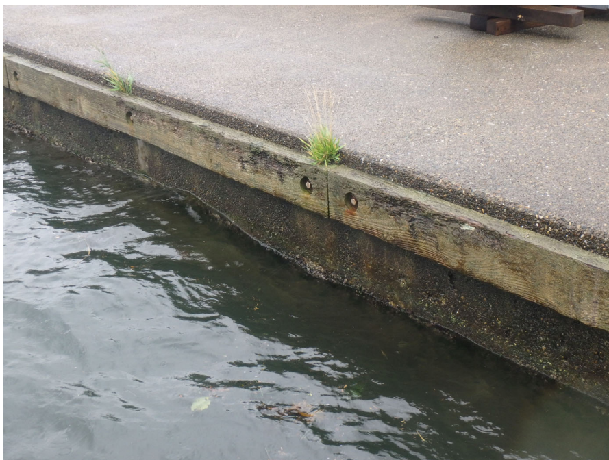
Photo 10. Worn timber rubboards with vegetation.
