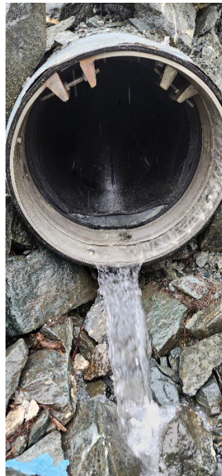
Figure 4 Image of the installed and functioning check valve – Meander at Northland Outfall
