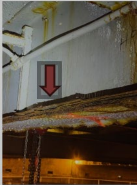
2. Corrosion at primary structural I-beam. Note significant corrosion at bottom flange causing delamination of the steel.
