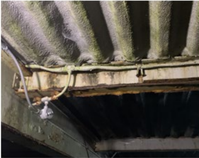
7. Underside view of metal roof decking. Foam Insulation is saturated with water. Note Algae growth.
