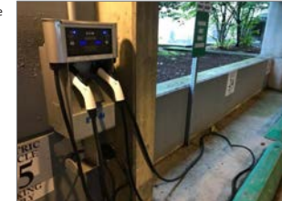
Marine Parking Garage EV Charging Station
