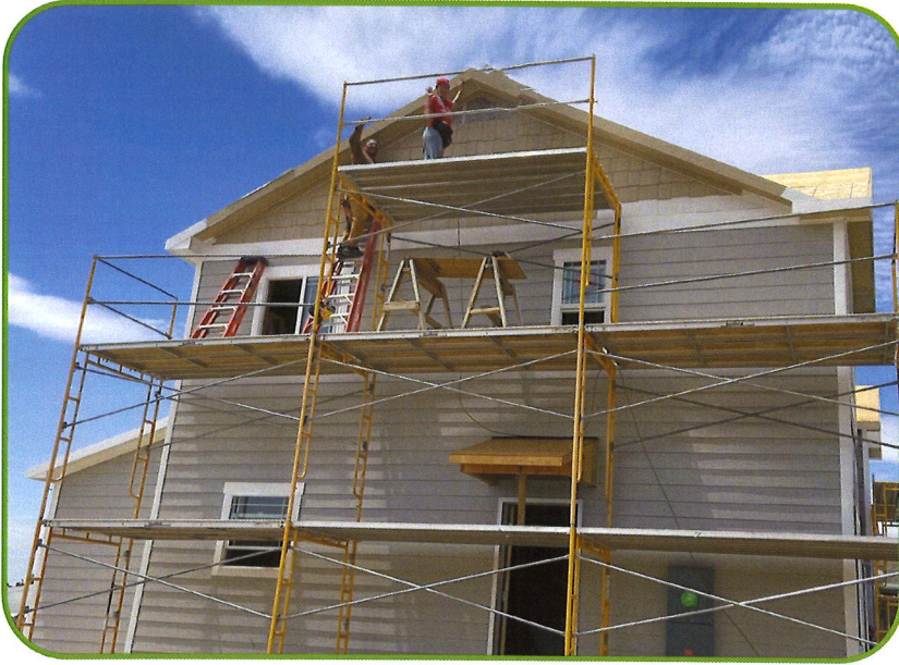
The Weld Trust staff, Rigo Rangel and Kristen Mullen, volunteering at a home build for Greeley-Weld Habitat for Humanity
