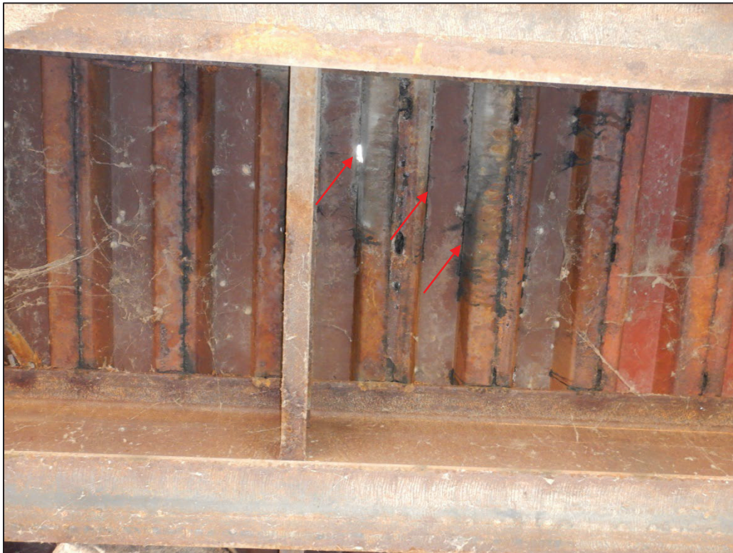
Hole and Cracking in Deck Flutes in Bay D
