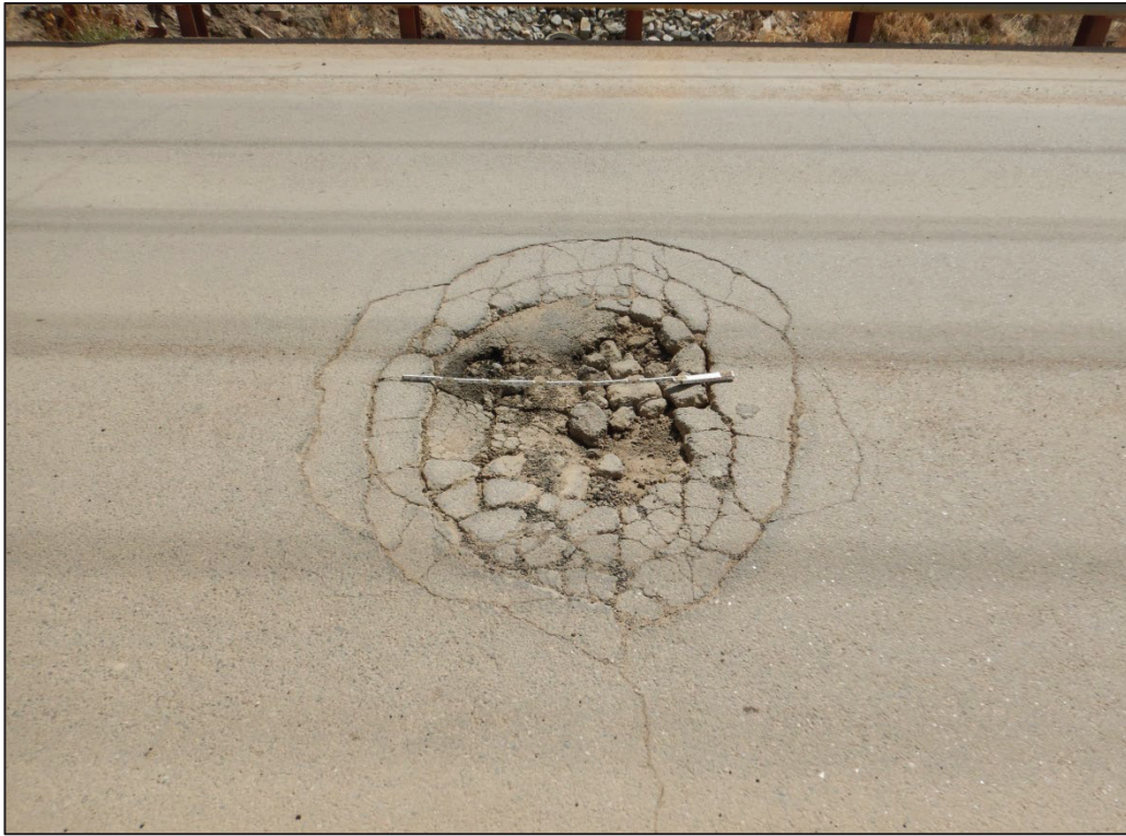
Full Depth Pothole and Broken-up Asphalt on Deck
