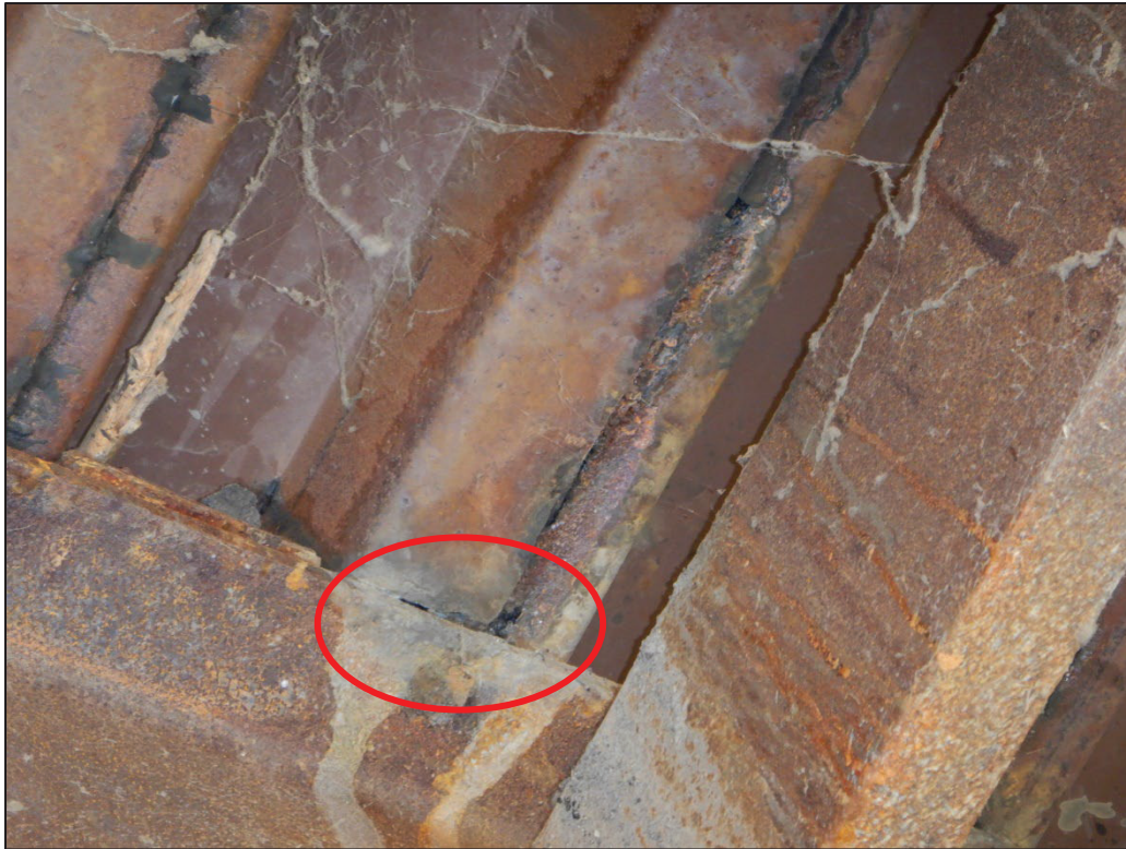
Cracking Across Deck Flute Adjacent to Hole above Girder D
