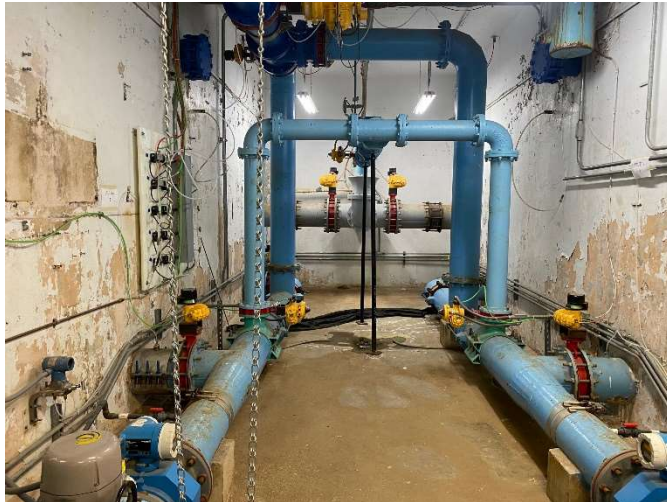
Photo: JWTP Existing Filter Pipe Gallery
