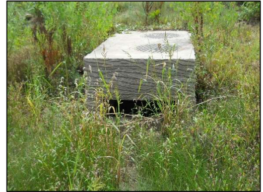
Water Quality Outlet Structure
