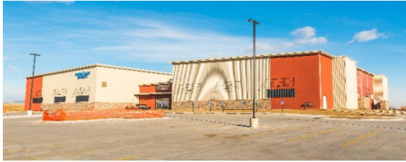
Figure 2-33 Unacceptable Metal Panel
