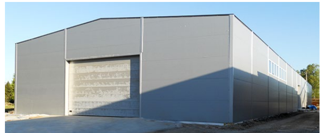
Figure 2-38 Unacceptable Metal Panel
