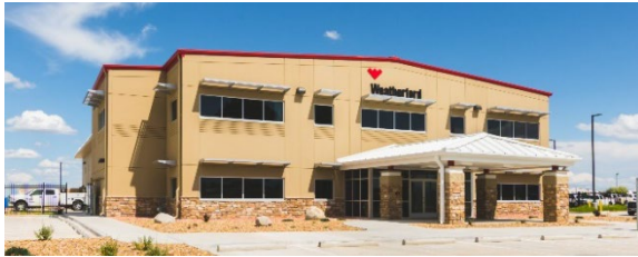
Figure 2-35 Unacceptable Metal Panel
