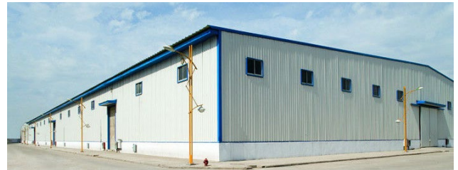
Figure 2-36 Unacceptable Metal Panel
