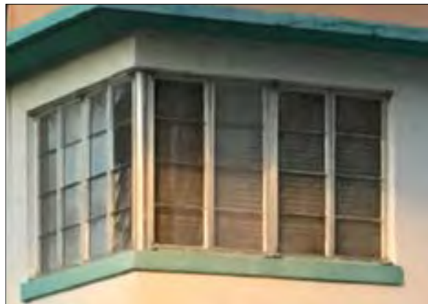
GROUPED CASEMENT WINDOWS WRAPPING A CORNER WITH A PIPE COLUMN AT THE EDGE
