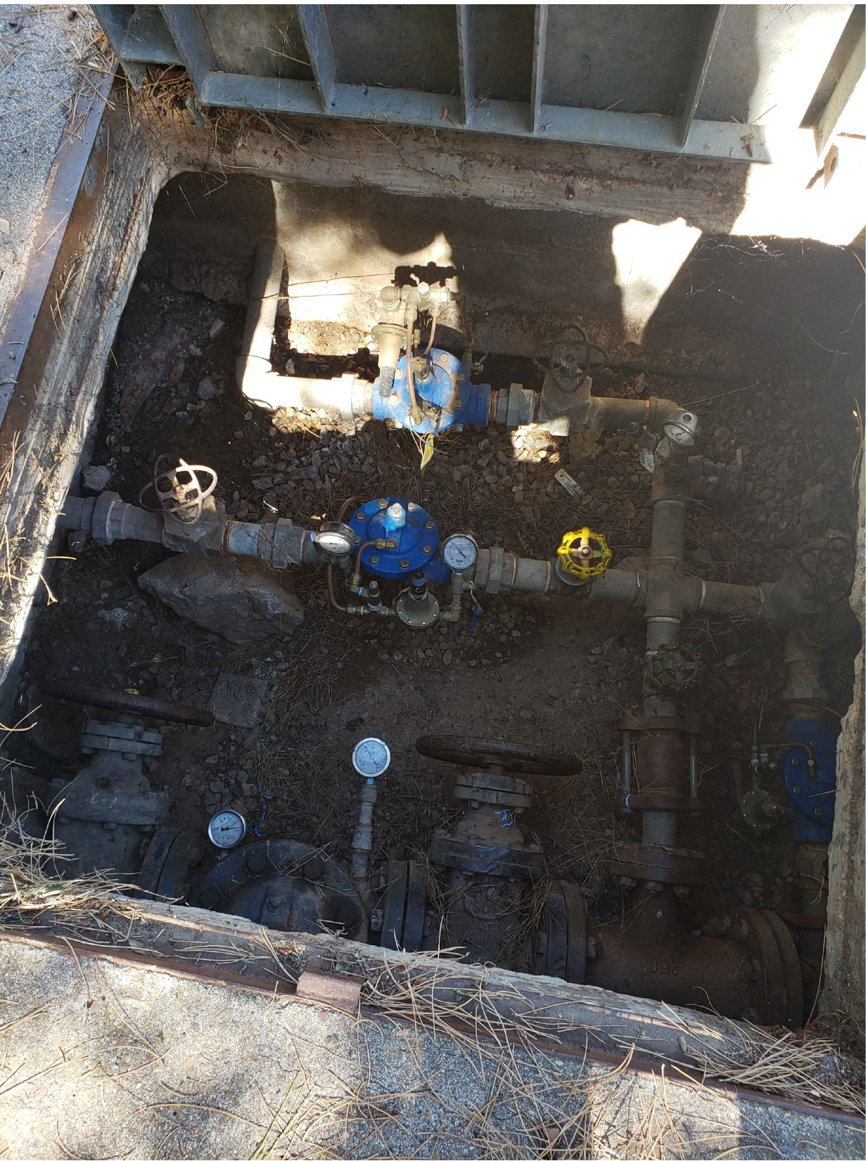
PHOTO OF EXISTING REGULATOR
