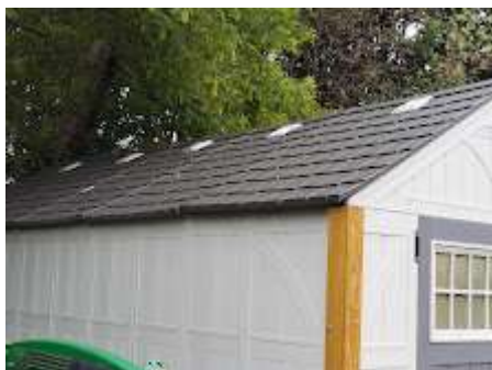
CR hail damage 2023 plastic roof and skylights.jpg 4643K
