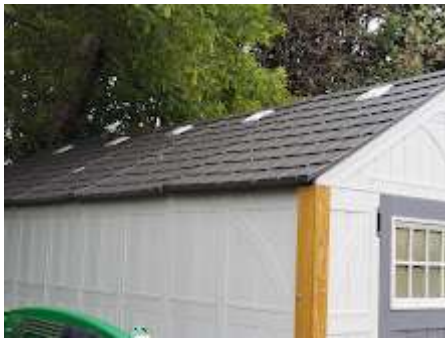
CR hail damage 2023 plastic roof and skylights.jpg 4643K
