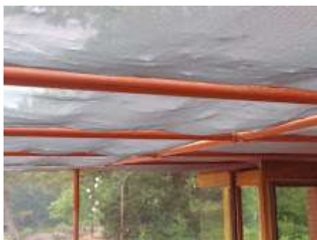
CR hail damage 2023 RP copper screen.jpg 5601K
