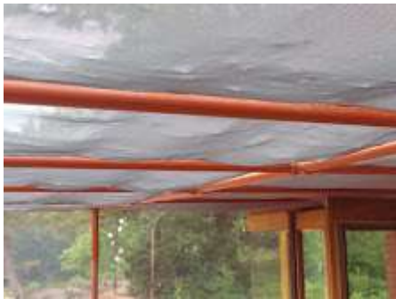
CR hail damage 2023 RP copper screen.jpg 5601K
