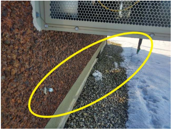
HVAC Ground Missing Before
