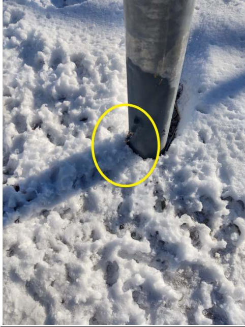
Ice Bridge Post #2 Ground Missing
