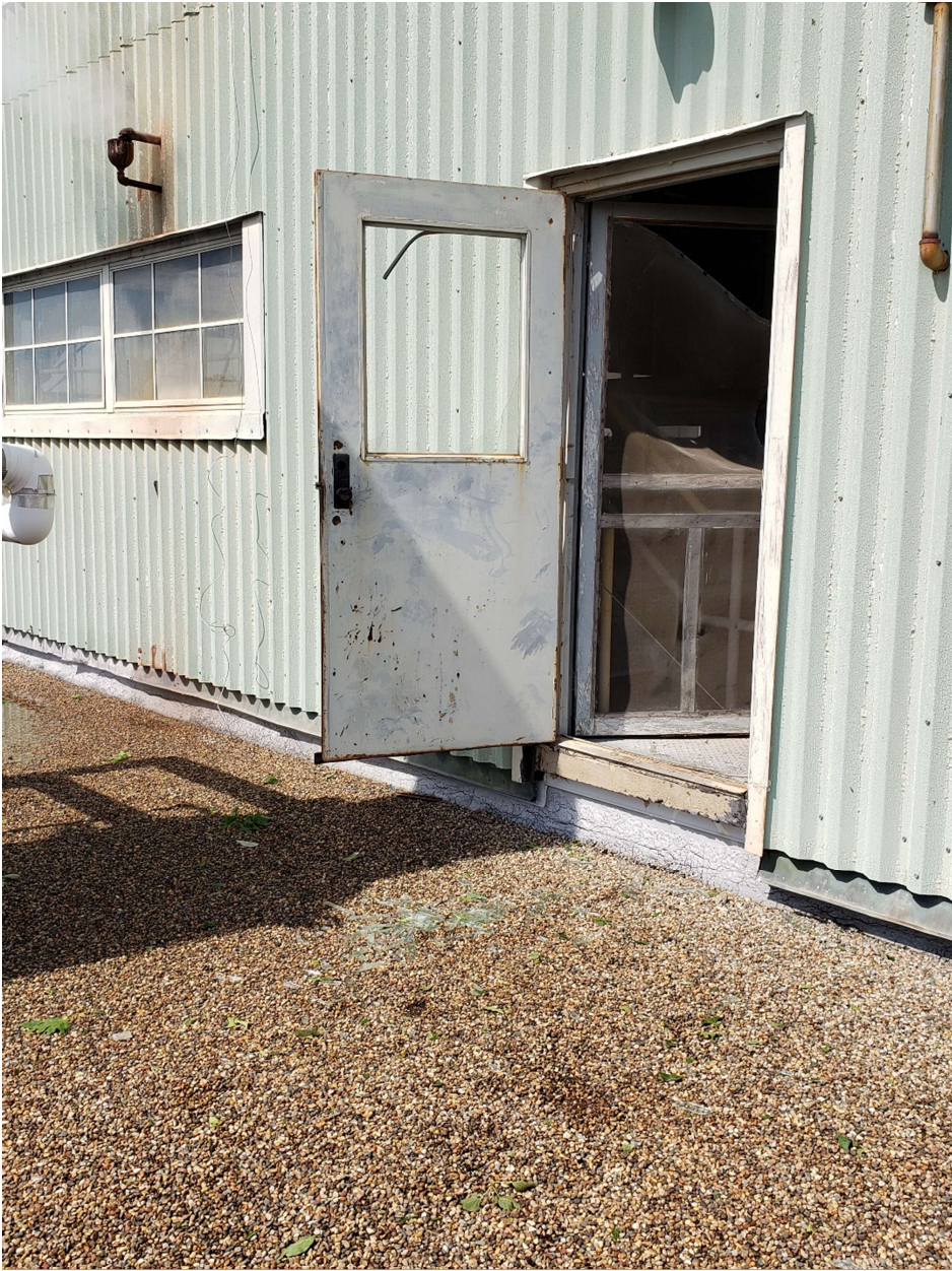
Glass in door has shattered
