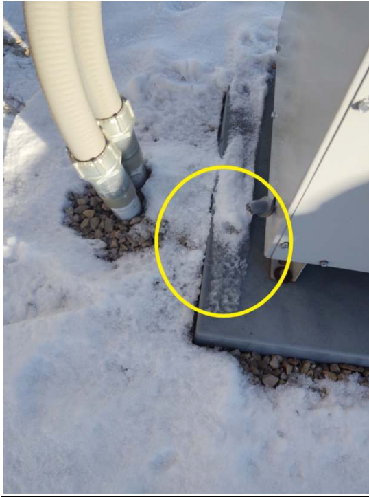
Isolation Transformer Ground Missing
