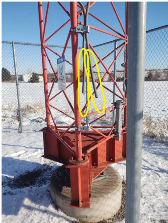
Tower Ground Bar Grounding Cables Missing
