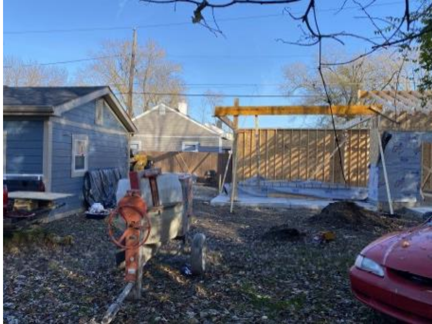
Photo 7: Unpermitted Garage Viewed from East (November 2025)
