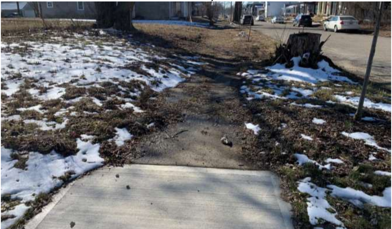
Photo of the sidewalk conditions in front of the property.
