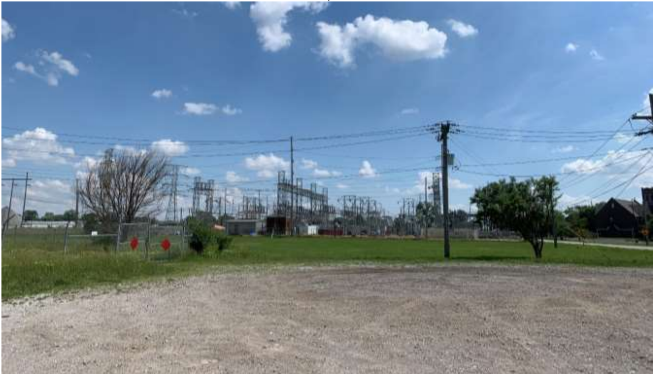
Photo of the IPL substation south of the site.
