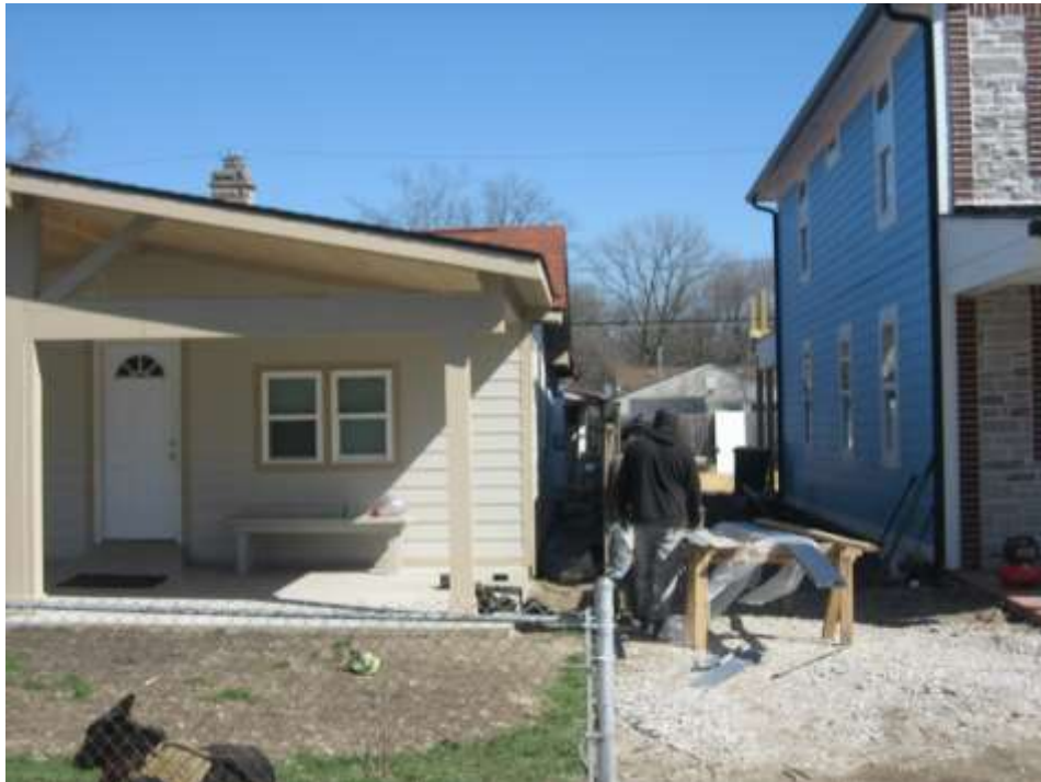
Photo of the existing single-family dwelling zzero-foot south side setback, looking east.
