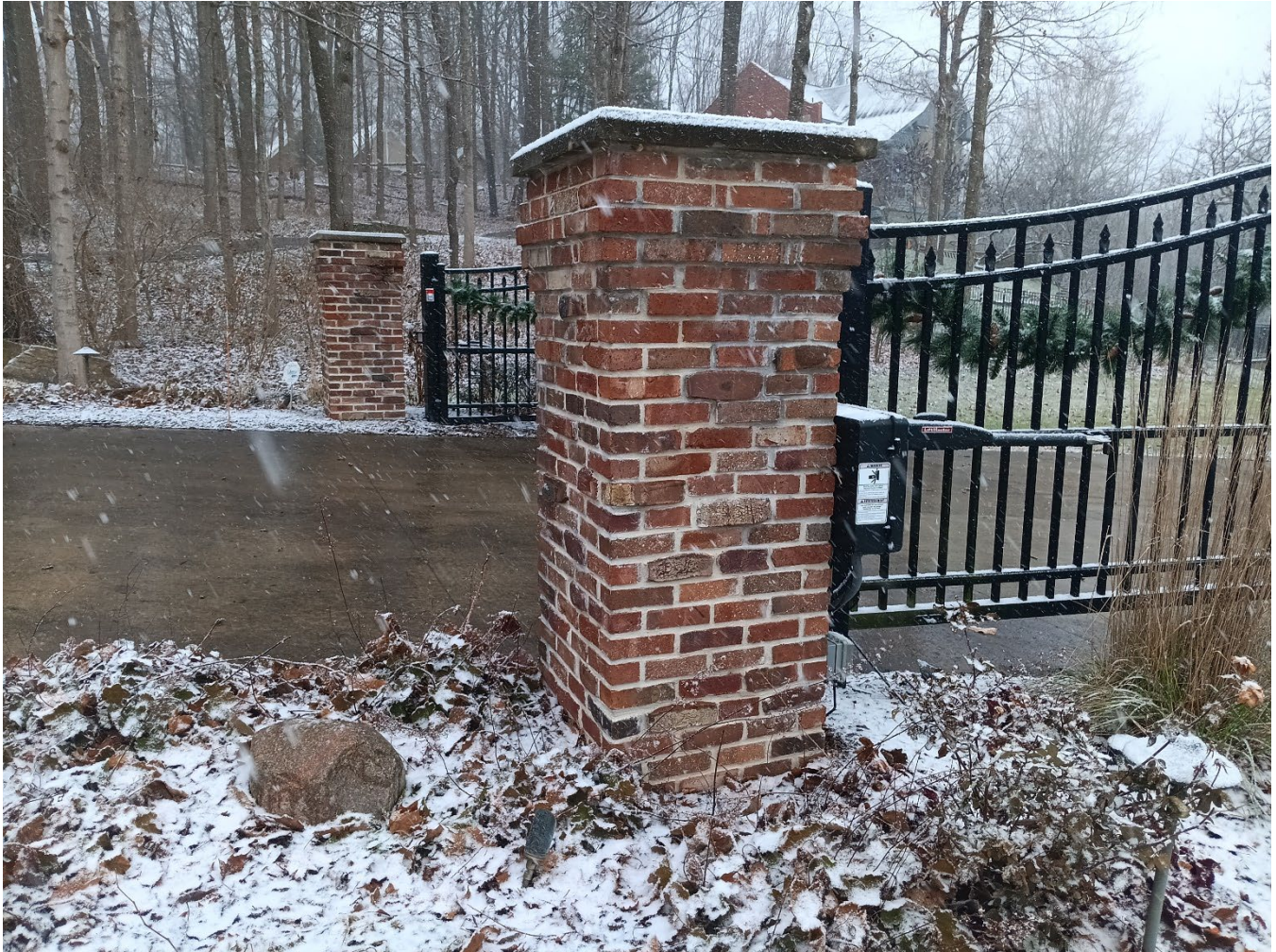
Exhibit 7: West Driveway Entrance, the bricks of the fence will match the bricks of these columns.
