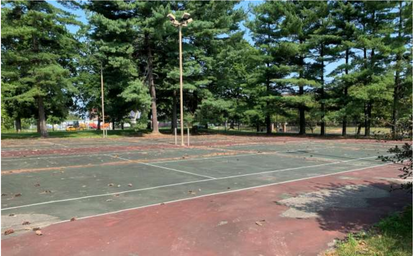
Close-up of the condition of the existing tennis courts to be removed.
