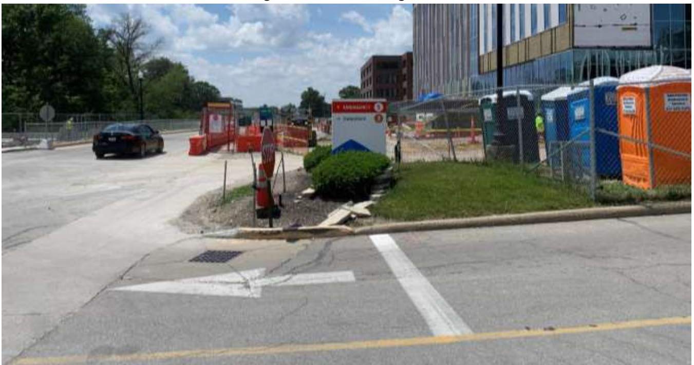
E08 to be replaced along Kate Knox Drive.
