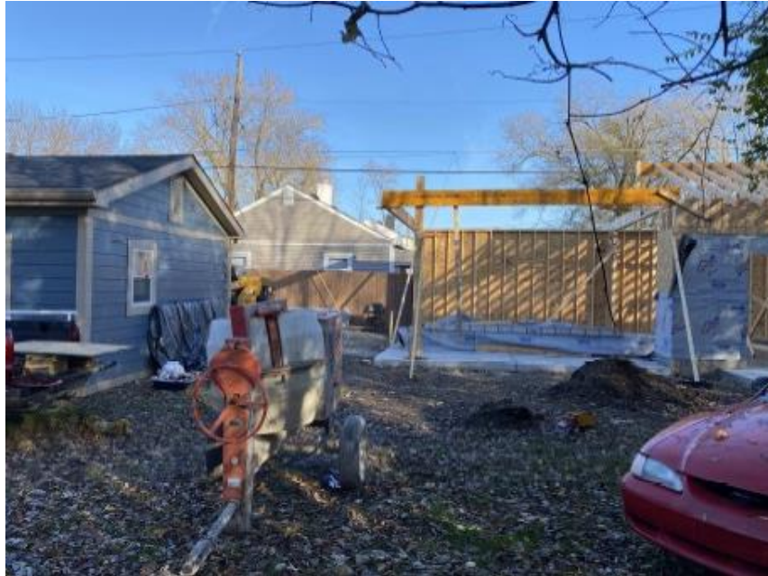
Photo 7: Unpermitted Garage Viewed from East (November 2025)
