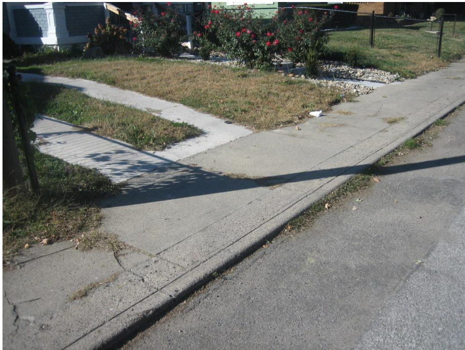
Photo 2 - Subject property existing low rise curb, that is driven over to access the non-permitted driveway, looking northwest.
