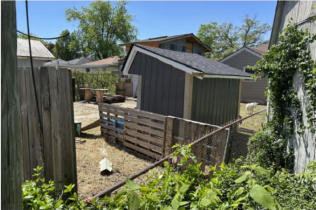
Photo 4: A BNS inspector's photo showing the shed encroaching into the side yard setback. Notice the open space where the shed could be moved to comply with setback standards. A goat can be seen in the photograph as well.
