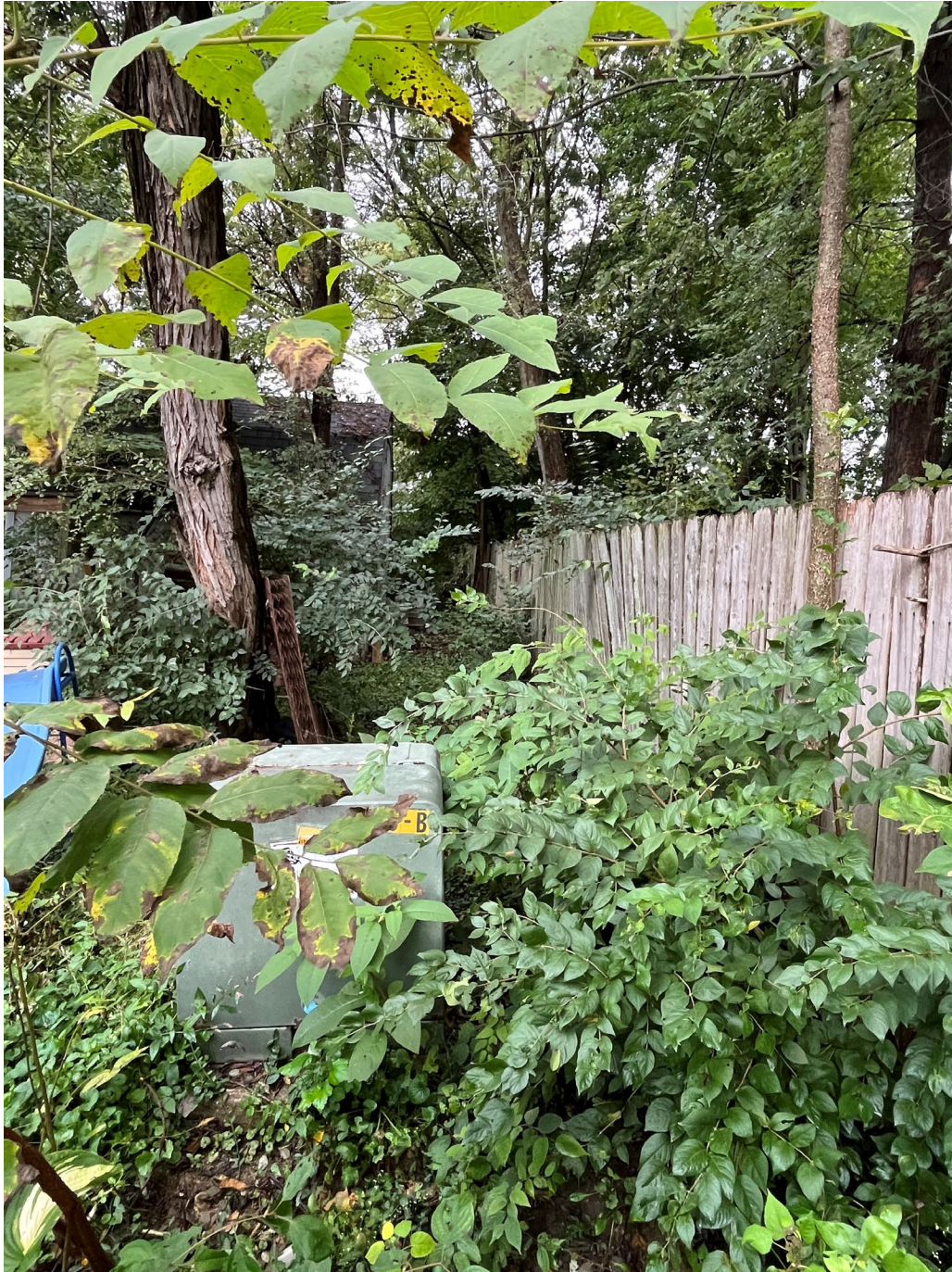
Electric utility box with shed in background
