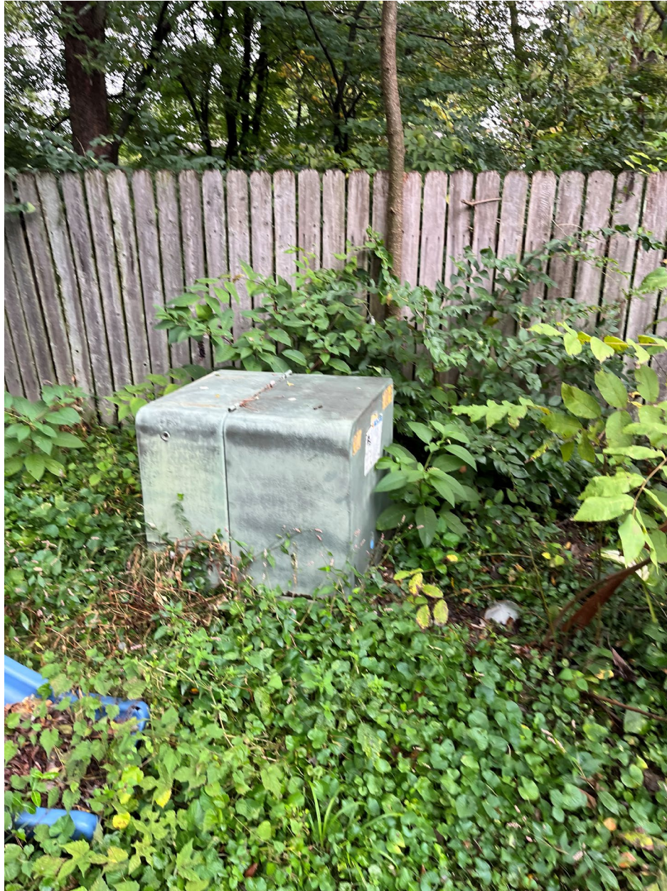
Electric utility box
