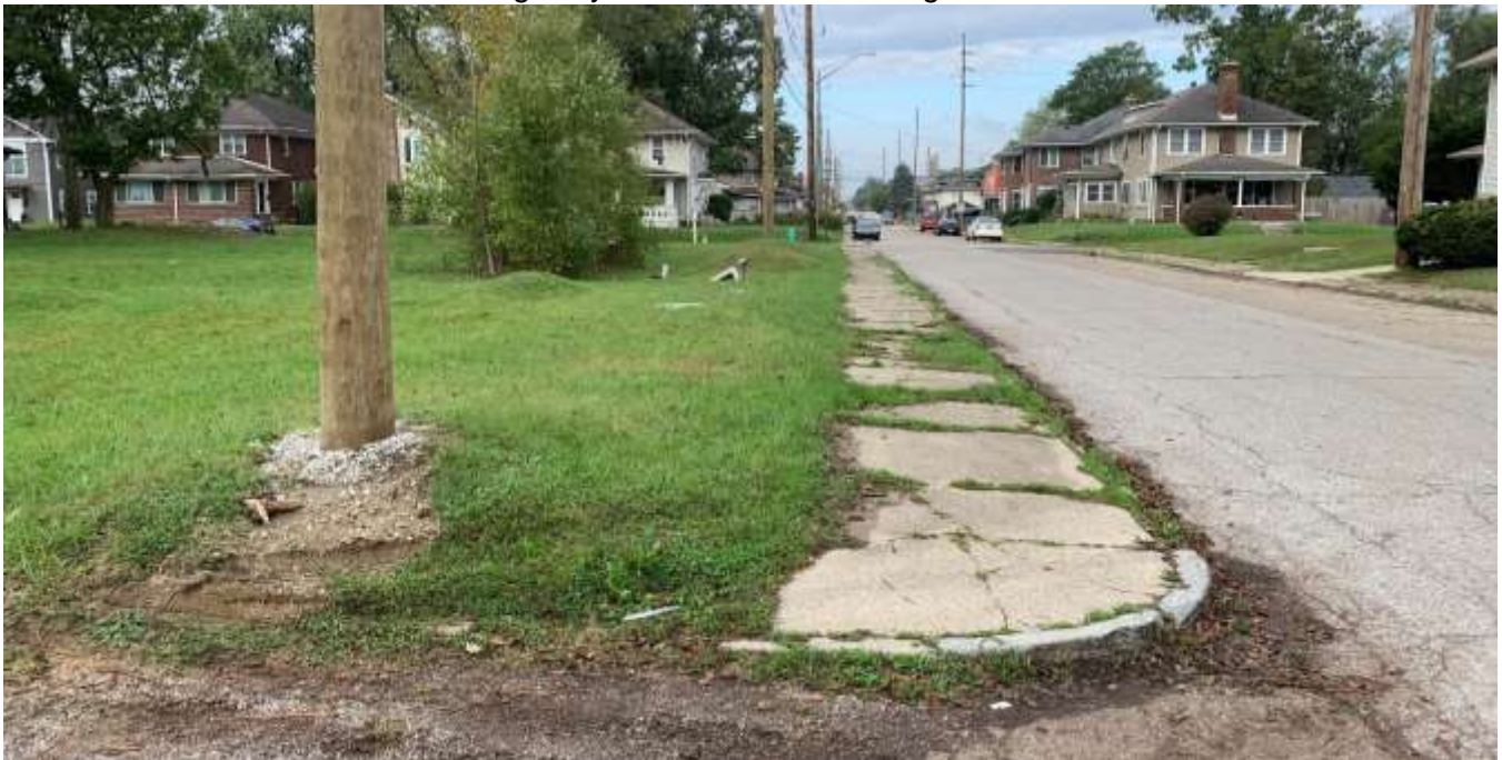
Photo of the sidewalk along 34 th Street looking west from the alley.
