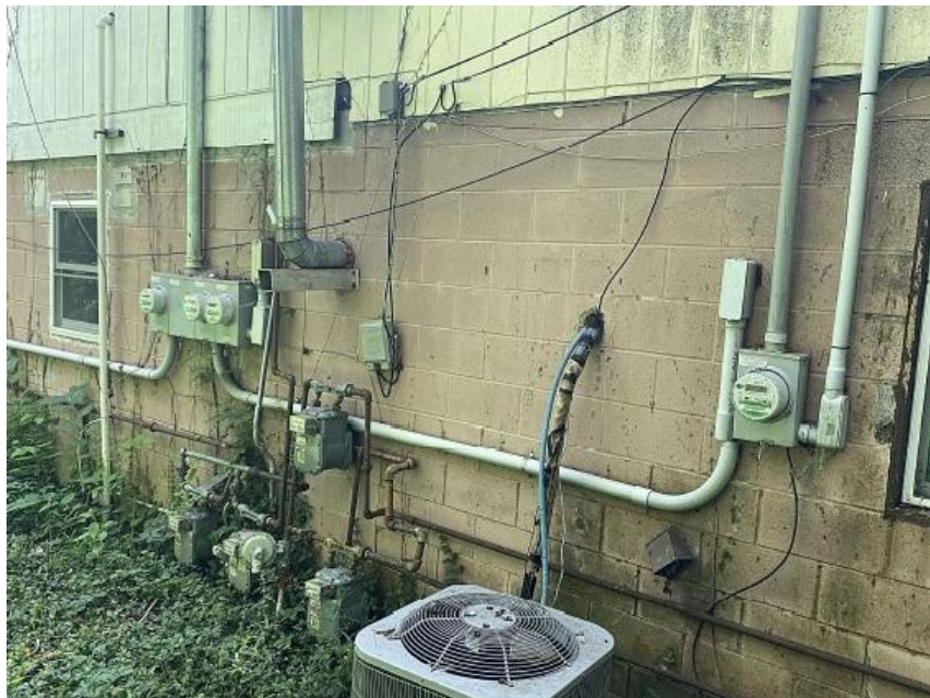
Photo 6: Multiple Power Meters on Multi-Family Building
