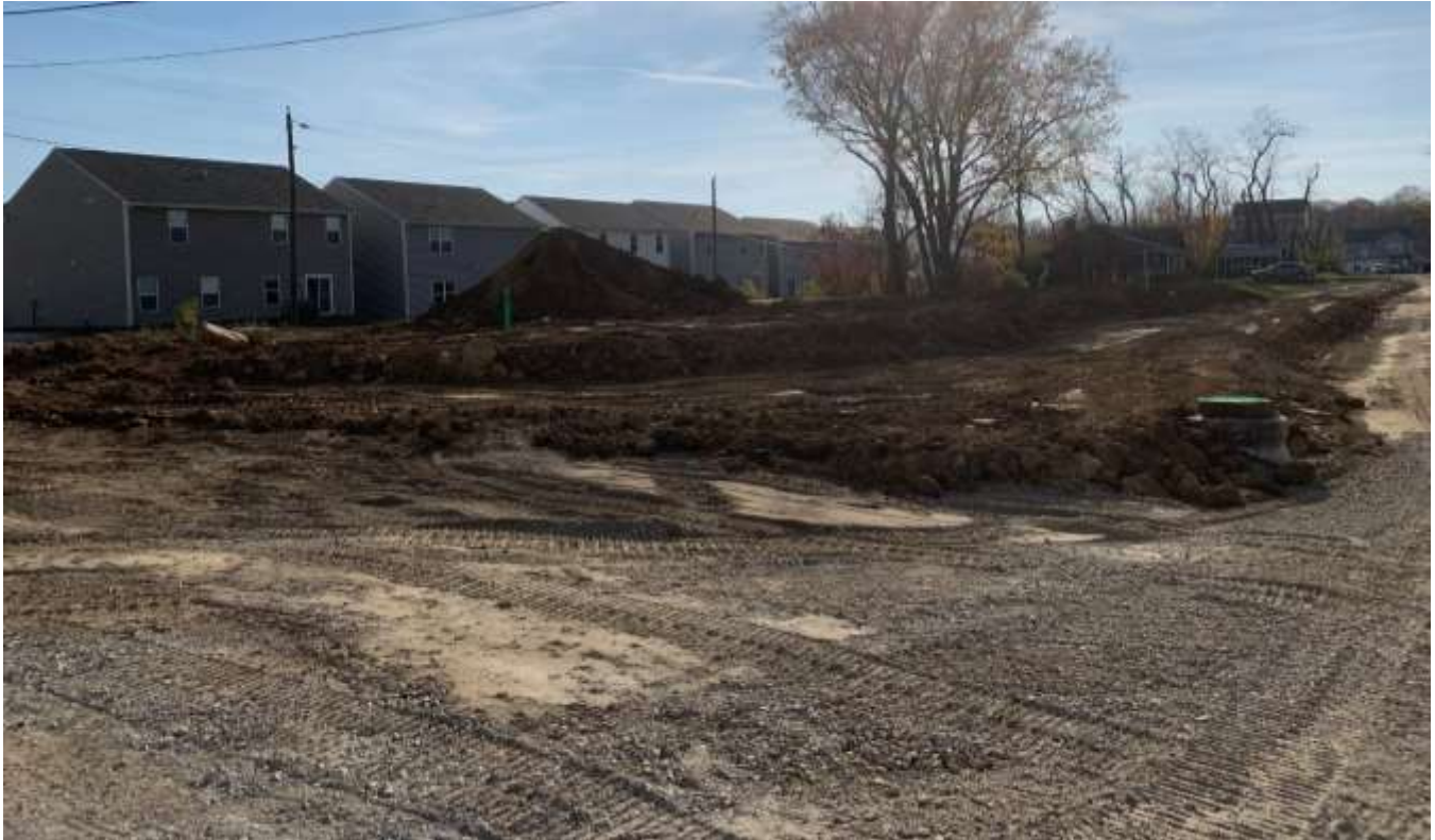
Photo looking southwest along the south side of Moonstone Street from Amethyst Avenue.
