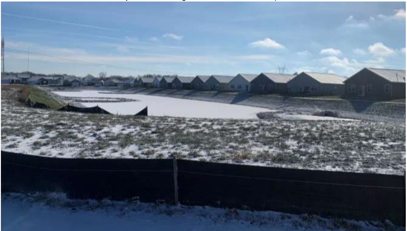
Photo of the subject site looking southeast at the D5-II portion of the site. |
