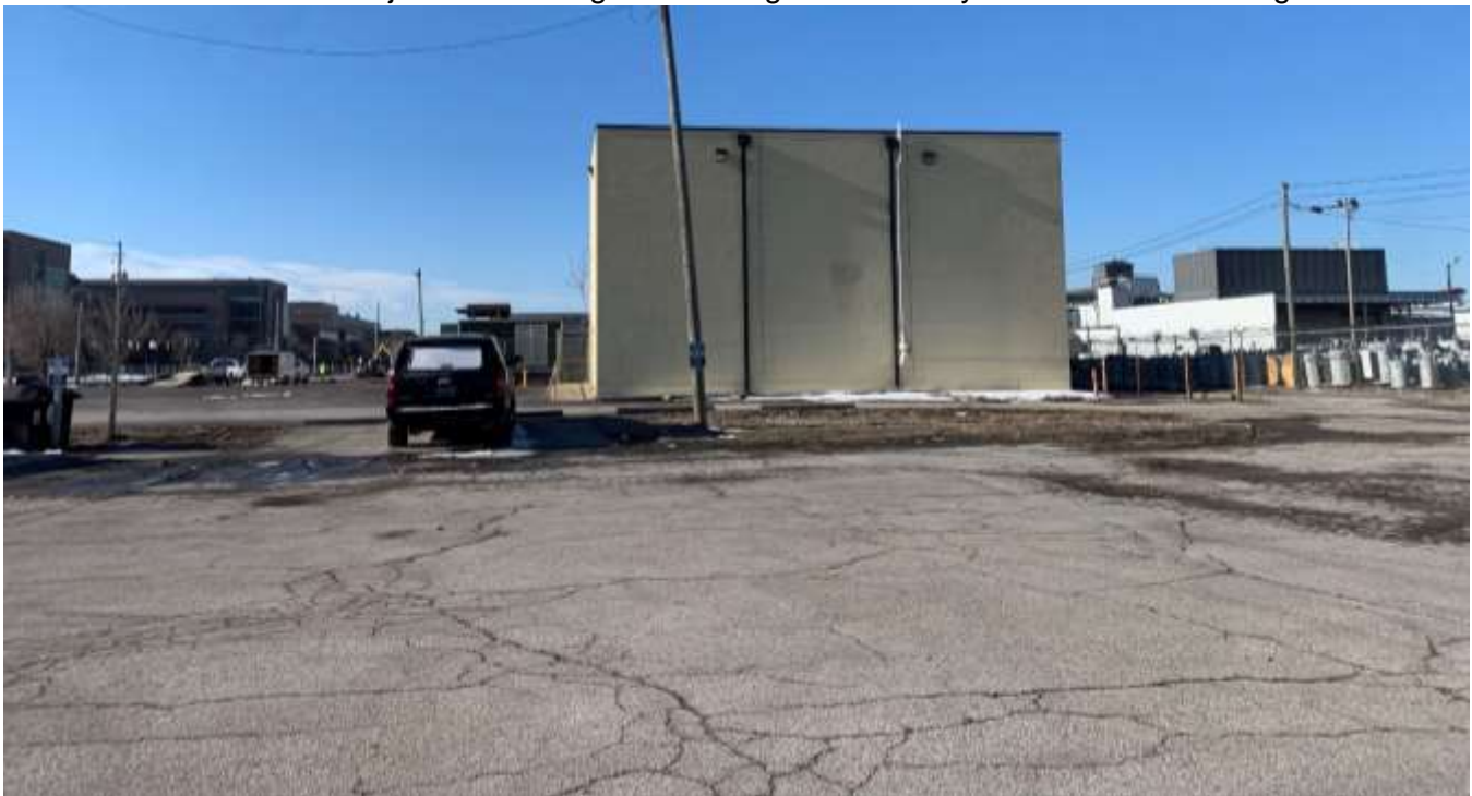
Photo of the existing building looking south from the property to the north.
