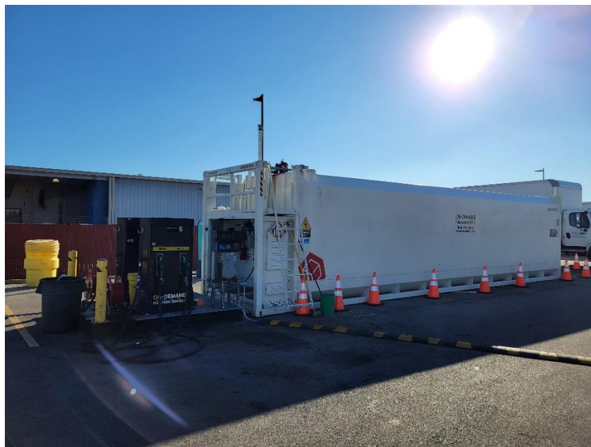
Photo 6: Temporary Fueling Station at Northeast of Property
