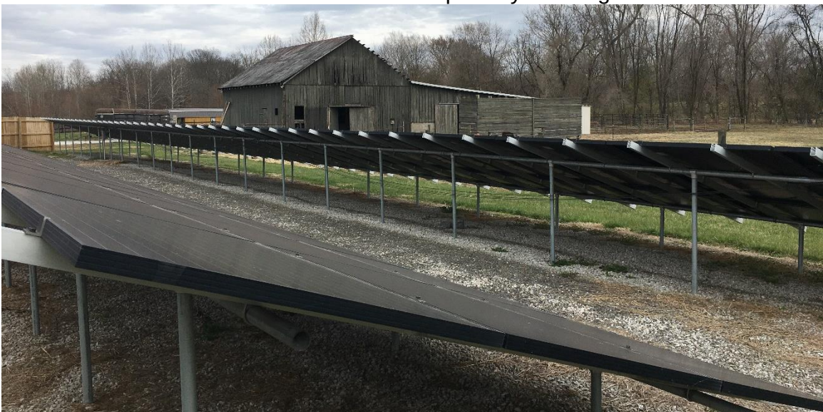
Solar panels on side/rear yard, looking east
