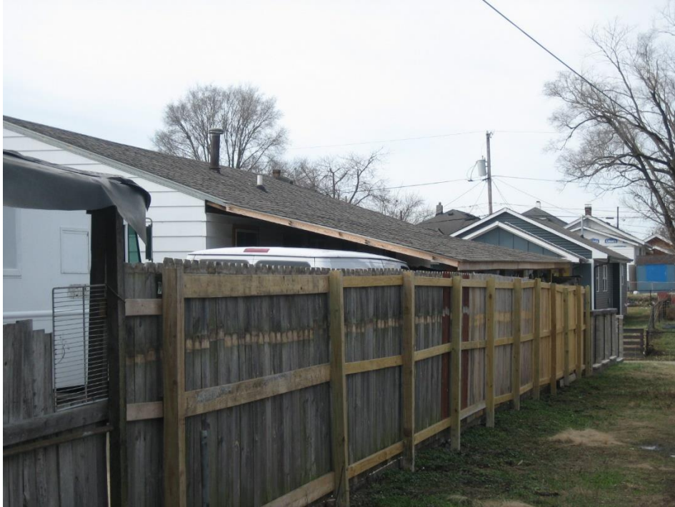
Photo 3- Subject property attached covered porch with zero-foot north side yard setback, looking west.
