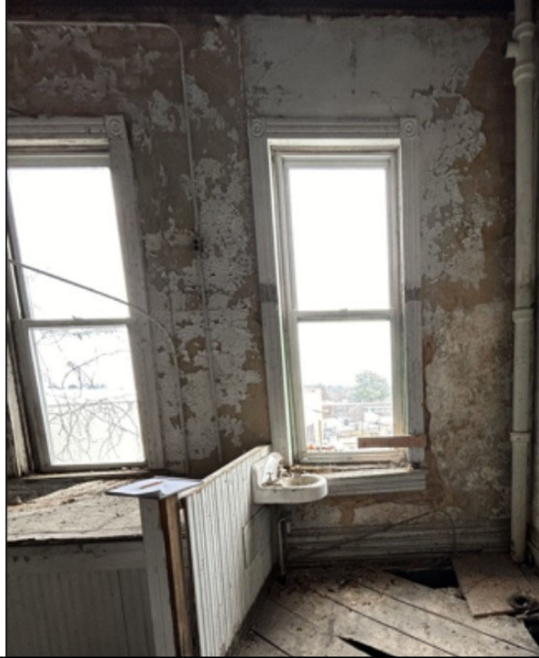
Applicant provided imagery of damaged windows
