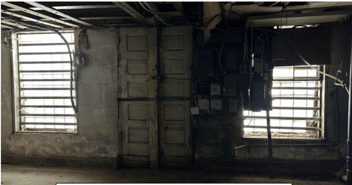
Applicant provided imagery of damaged windows
