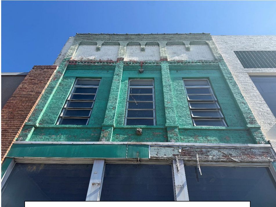
Upper facade detail showing damage
