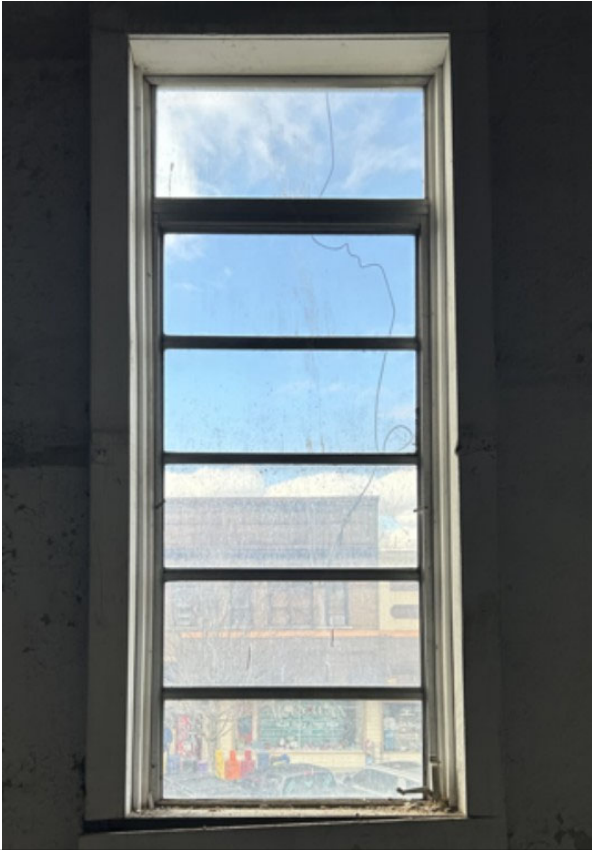
Applicant provided imagery of damaged windows
