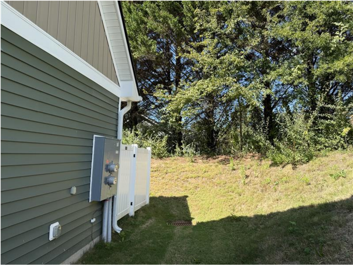
Photo 2: Northern corner of building encroaching into setback.
