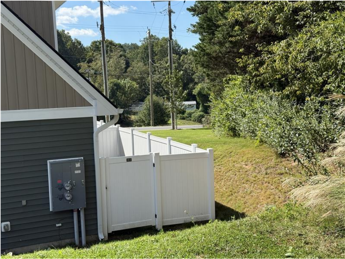
Photo 3: View north west of corner of building encroaching into setback.
