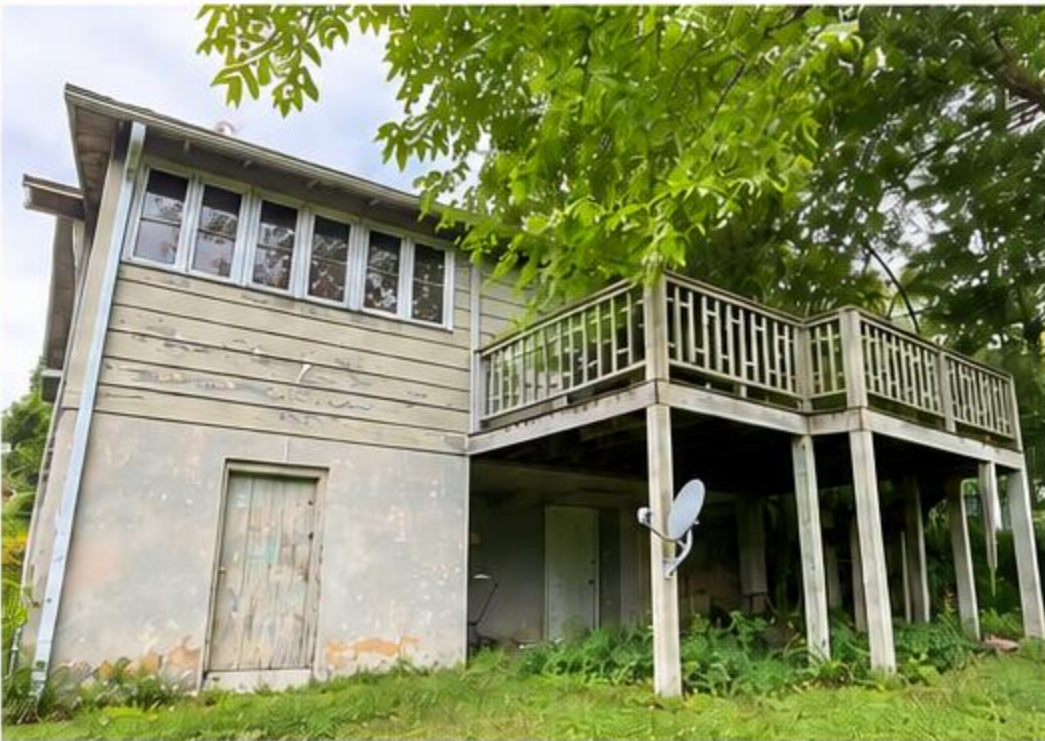
Existing rear elevation showing deteriorated deck.
