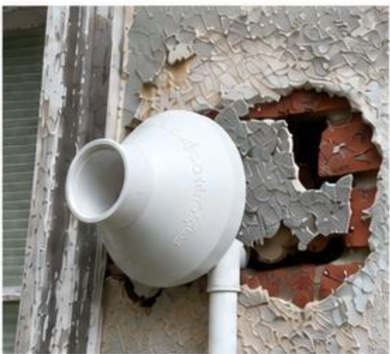
EXISTING CONDITION DAMAGED STUCCO / EXPOSED MASONRY
