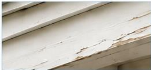
Wood Fascia Repair or replace in kind.
