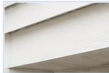
Wood Fascia Repair or replace in kind.
