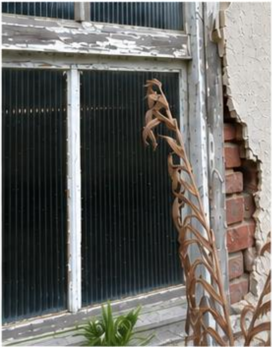
EXISTING CONDITION DETERIORATED STUCCO / EXPOSED MASONRY
