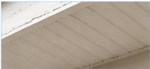
Wood Soffit Repair or replace in kind.
