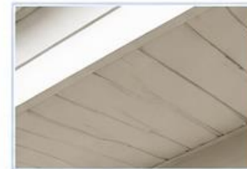
Wood Soffit Repair or replace in kind.
