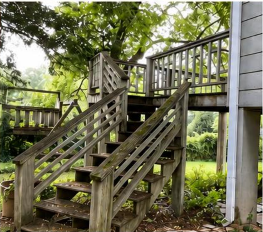
Existing deck and stairs with deterioration.
