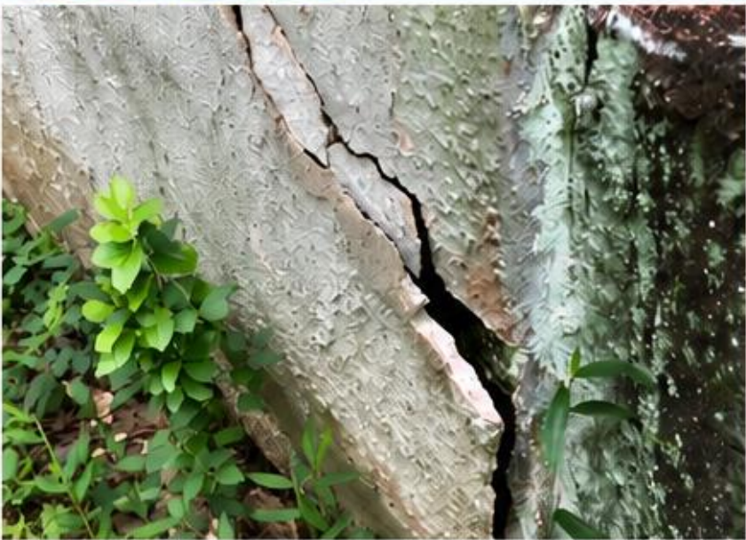
Example of concrete cracking and deterioration on side steps contributing to water infiltration at the foundation wall.
