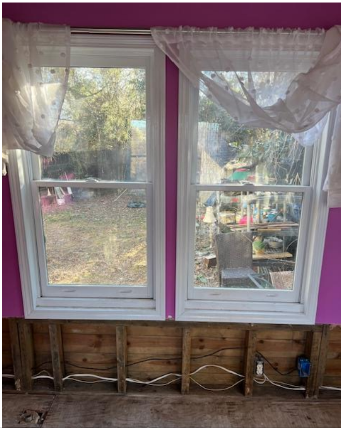
Interior photos of windows proposed to be removed and replaced with double doors.
