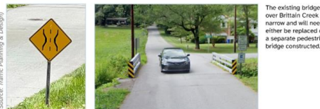
The existing bridge over Brittain Creek is narrow and will need to either be replaced or a separate pedestrian bridge constructed.
