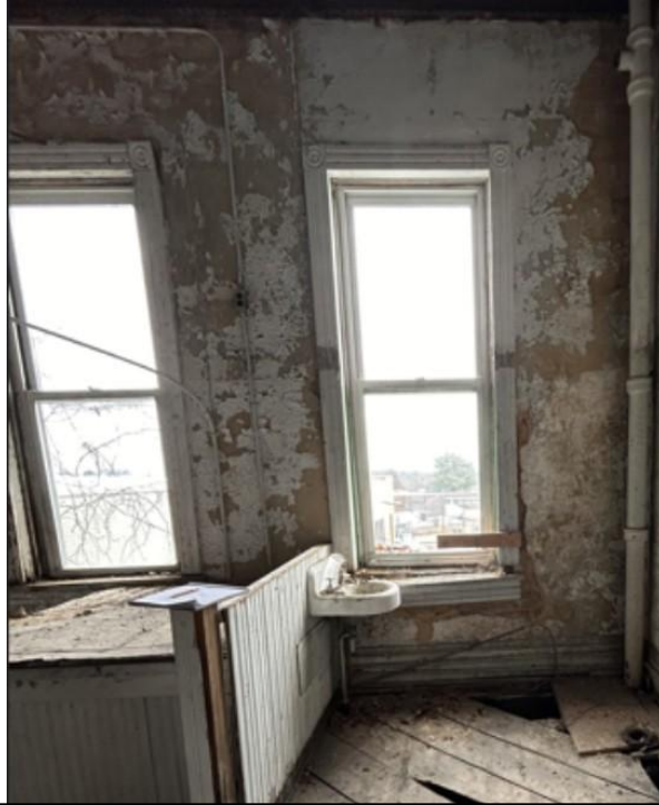
Applicant provided imagery of damaged windows
