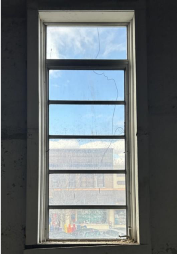
Applicant provided imagery of damaged windows
